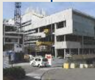
→ 2008 – New Zealand’s first PRESSS (Precast Seismic Structural System) building – the Alan MacDiarmid building at the Victoria University of Wellington features BBR CONA tendons in an innovative damage-resistant design application. NZ
