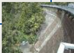
➔ 1992-93 – Installation of BBR CONA rock anchors for Waitakere Dam, Auckland, New Zealand. NZ
