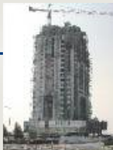
→ 2003 – Structural Systems’ first project in Qatar completed – the 24-storey Bilal Suites Tower in Doha. AUS
