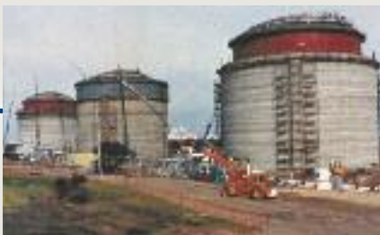
➔ 1990 – Design and construction of post-tensioning and slipform systems for three large LNG containment vessels in Kwinana, Western Australia. AUS
