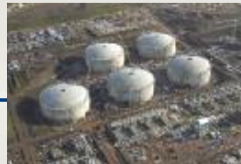
→ 2007 – Structural Systems UK’s largest project to date, the South Hook LNG tanks in Milford Haven in South Wales began. AUS
