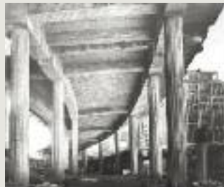
➔ 1974 – Shell Gully bridge structures – one of many bridge projects BBR Contech worked on in the 1970s during development of city and motorway infrastructure in Wellington. NZ
