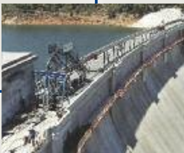
→ 2001 – World record set by Structural Systems in 2001 when they installed the largest permanent and restorable ground anchors at Canning Dam, Western Australia. AUS
