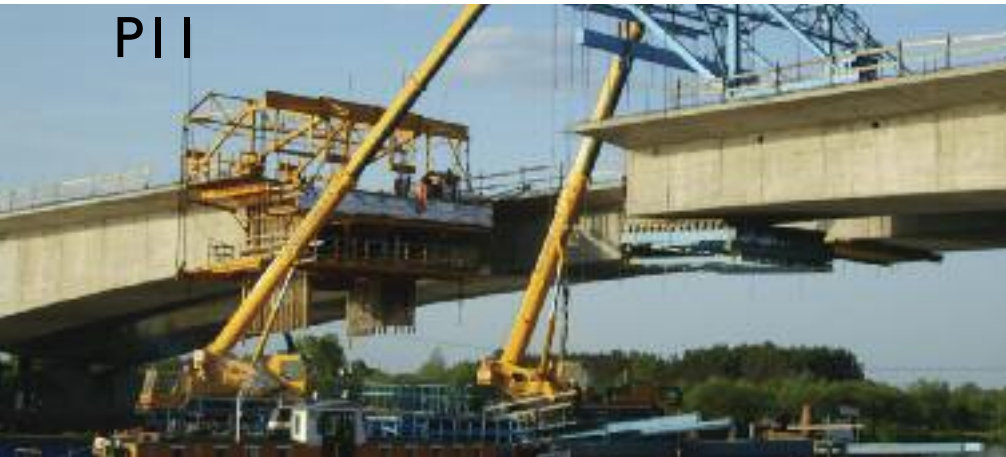
Part of a major pan-European highway, the new River Bug Bridge in northern eastern Poland was a complex free cantilever construction requiring two sets of form travelers.
