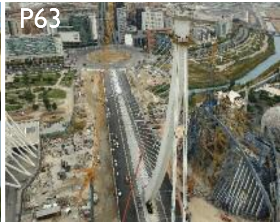
Calatrava's elegant new masterpiece in Spain provides not only a focal point for Valencia, but also reassurance that the very latest technology has been applied – the BBR HiAm CONA Stay Cable system.
