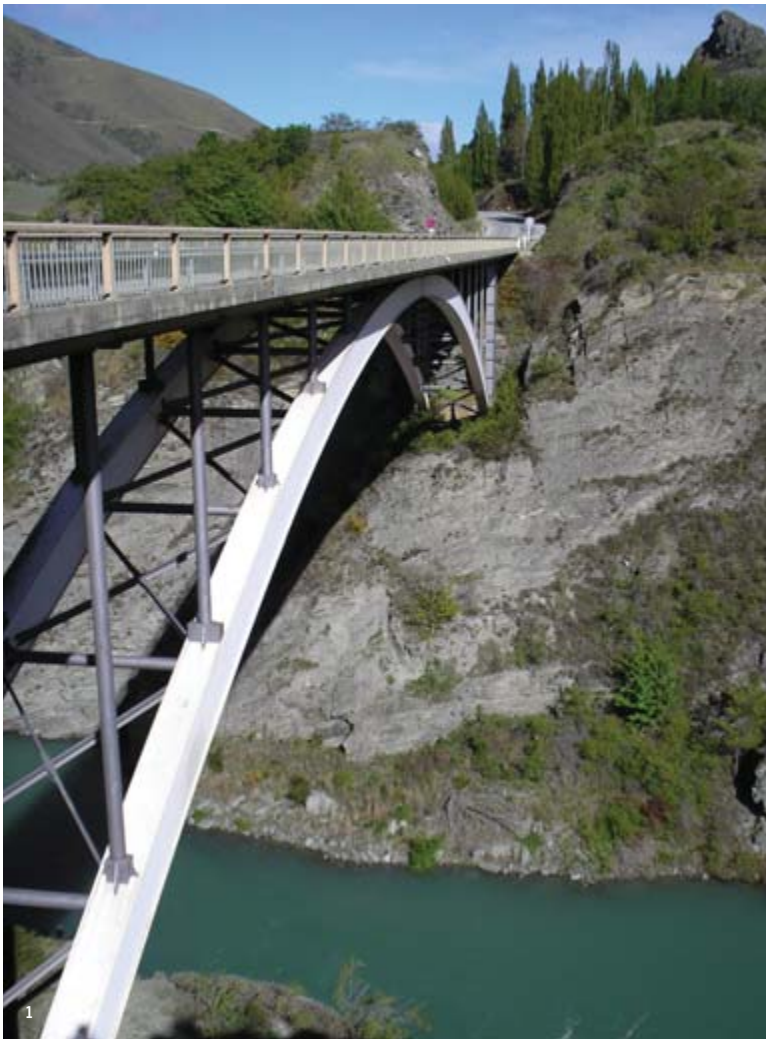
1 Seismic strengthening work was carried out by BBR Contech to the Kawarau Bridge, near Queenstown in New Zealand.
